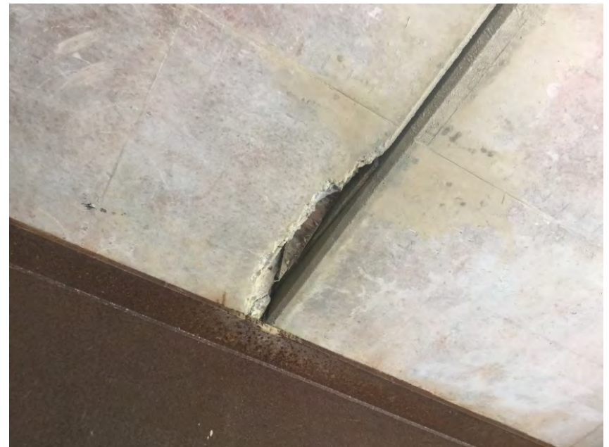
Damage to panel 1 right bank
