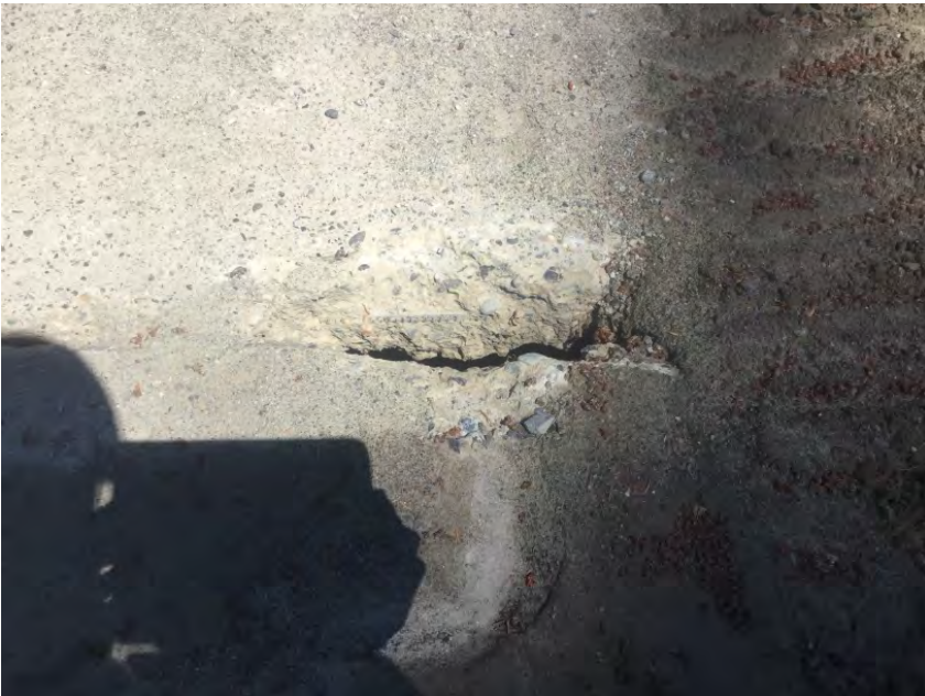
Deck damage right bank
