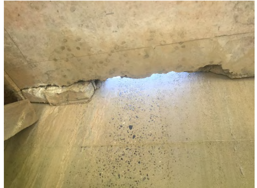
Damage to panel 1 right bank
