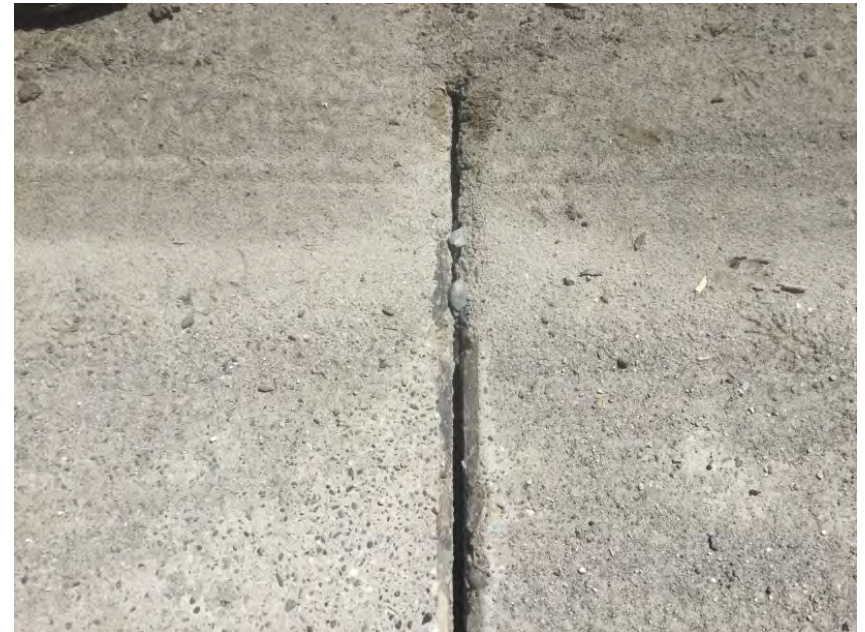
Deck joints missing rubber seals
