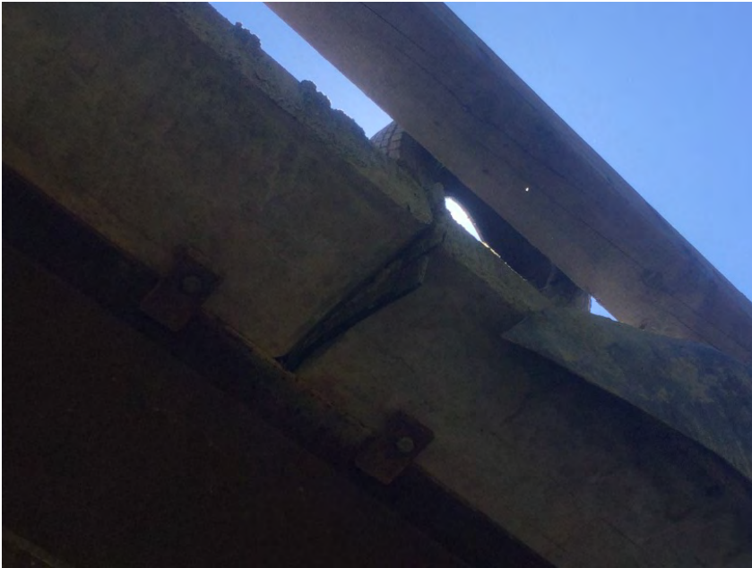
Deck seals failing
